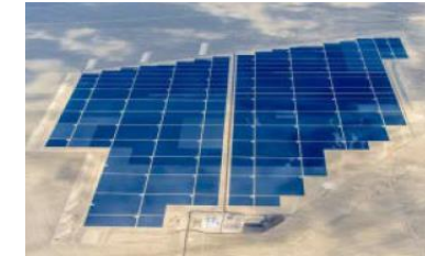
Utility Scale Solar
