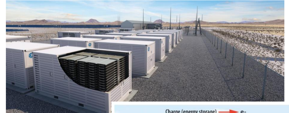
Source: GE ( https://www.ge.com/news/reports/leading-charge-battery-storage-sweeps-world-ge-finding-place-sun )
