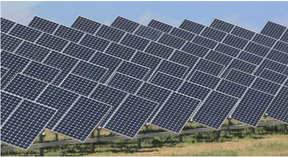
Xcel Energy’s Sandhill Solar Farm, CO.
