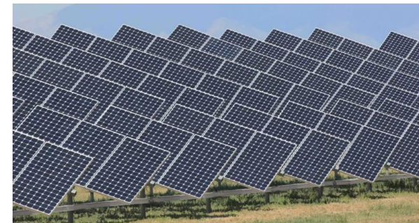
Xcel Energy's Sandhill Solar Farm, CO.
