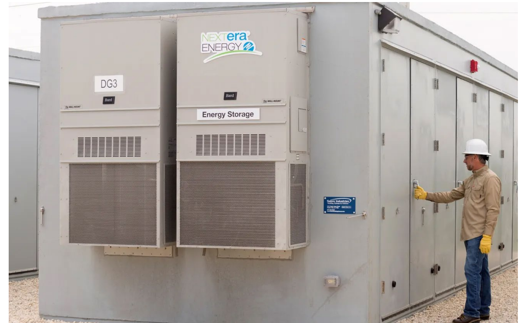
NextEra Energy battery storage. Source: EPE
